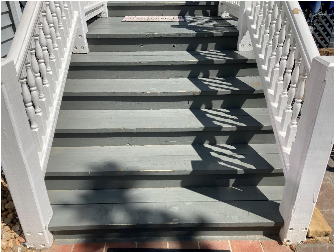
View of existing wooden stairs painted a dark blue color coming off the rear of the wooden one-story wraparound porch
