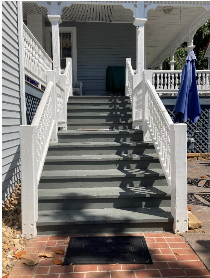
View of existing wooden stairs painted a dark blue color coming off the rear of the wooden one-story wraparound porch
