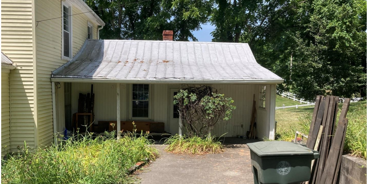
View of East elevation of rear ell extending North toward High Street
