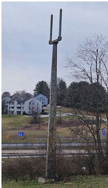
Missing Pylon Sign
