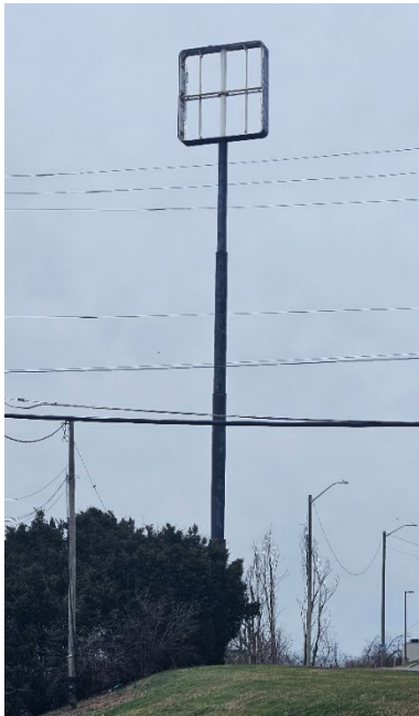
Missing Pylon Sign
