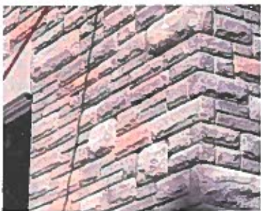
Dicketts Lane Elementary School, Abingdon, Virginia | Architect: HOK | Product: Citadel® | Color: Custom
